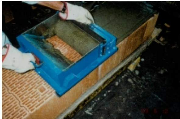
Picture 2: Apply of cover up thin layer mortar with a mortar box
