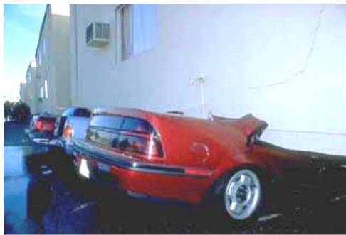
Figure 1: Northridge, ZDA, 1994; global failure because of the effect of soft storey mechanism
