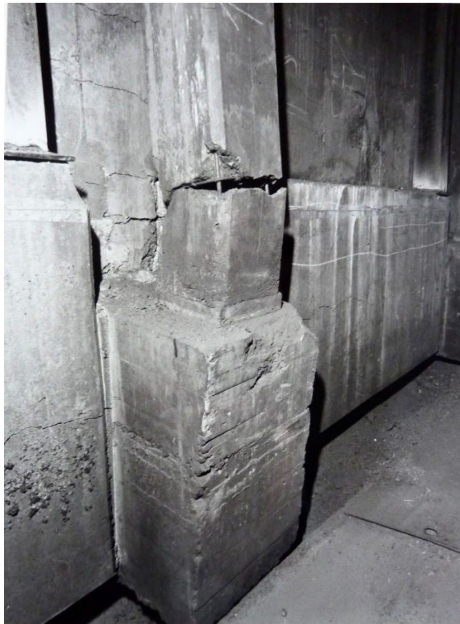
Fig. 5: Column with large crack, showing the small reinforcement (from [3])
