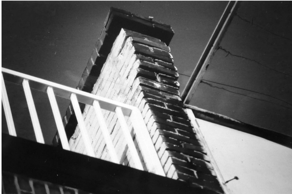
Fig. 1: Thermal permanent expansion of the partition wall
