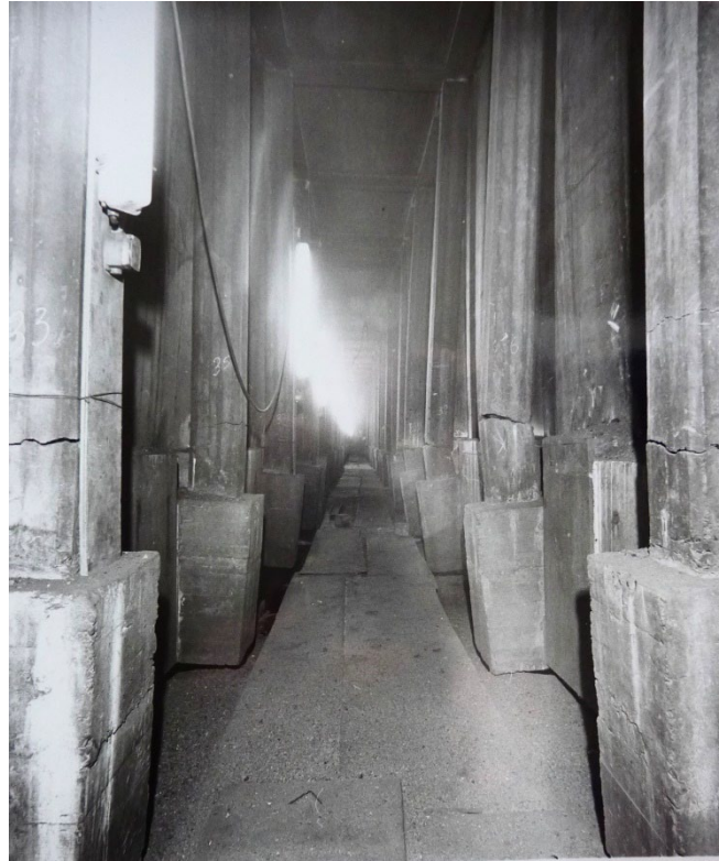
Fig. 4: Deformed concrete box and cracked columns (from [3])
