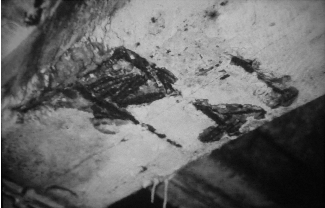
Fig. 9: Corrosion products on lower side of tension chord
