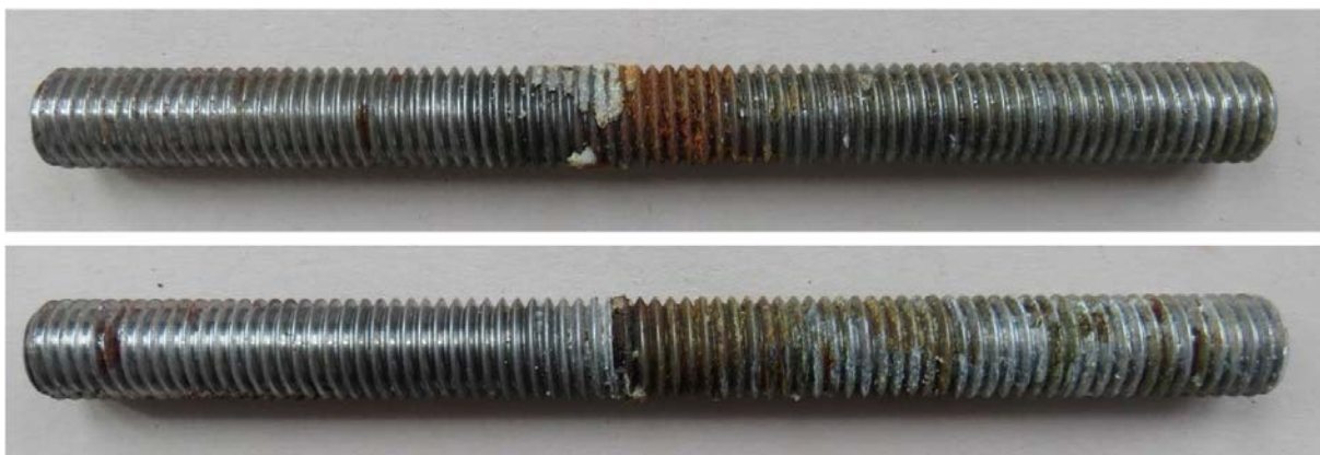
Fig. 3: Examples for the visual assessment of the threaded rods (vinyl ester based injection mortar) after 2 weeks (top) and 18 weeks (bottom) in artificial seawater
