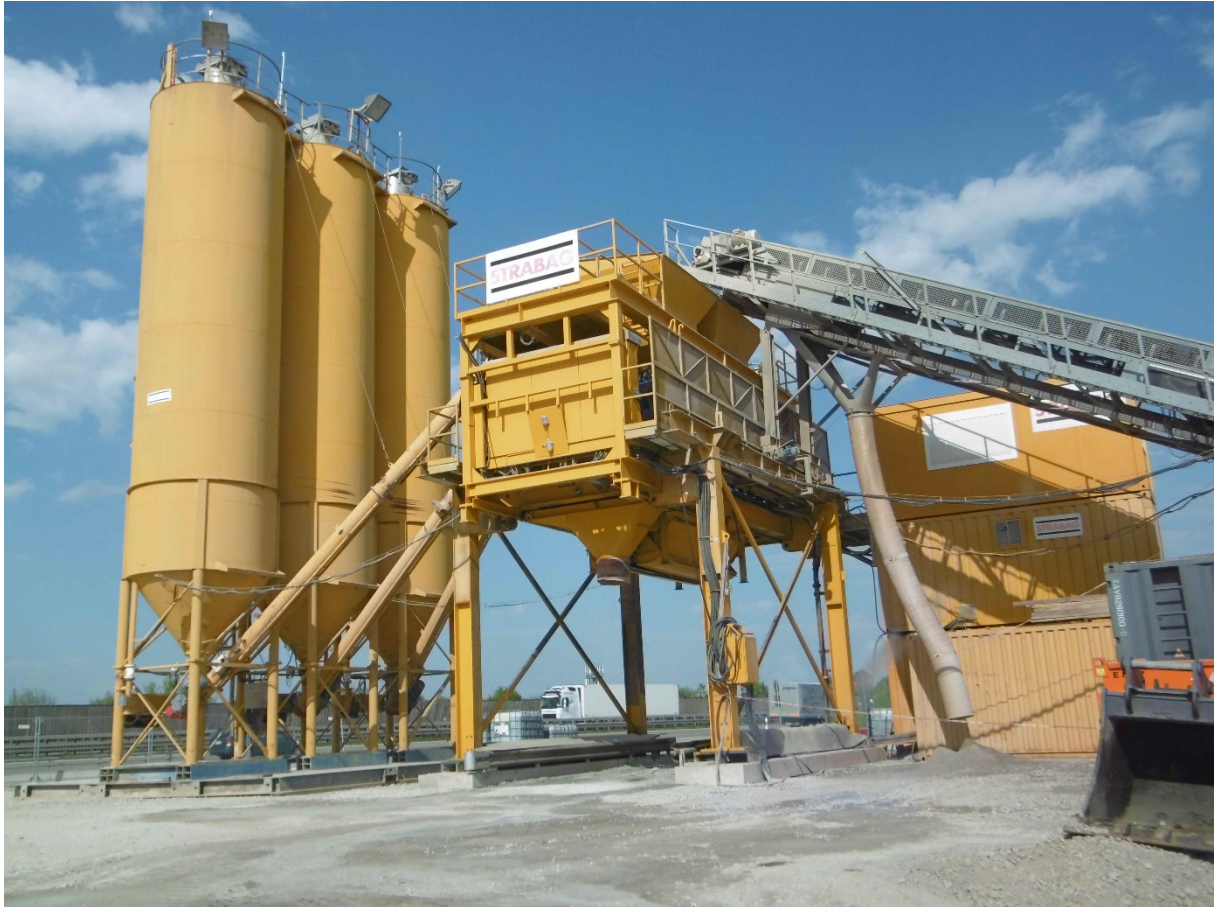
Fig. 5: Mobile batch mixing plant for the paver concrete and manually placed concrete
