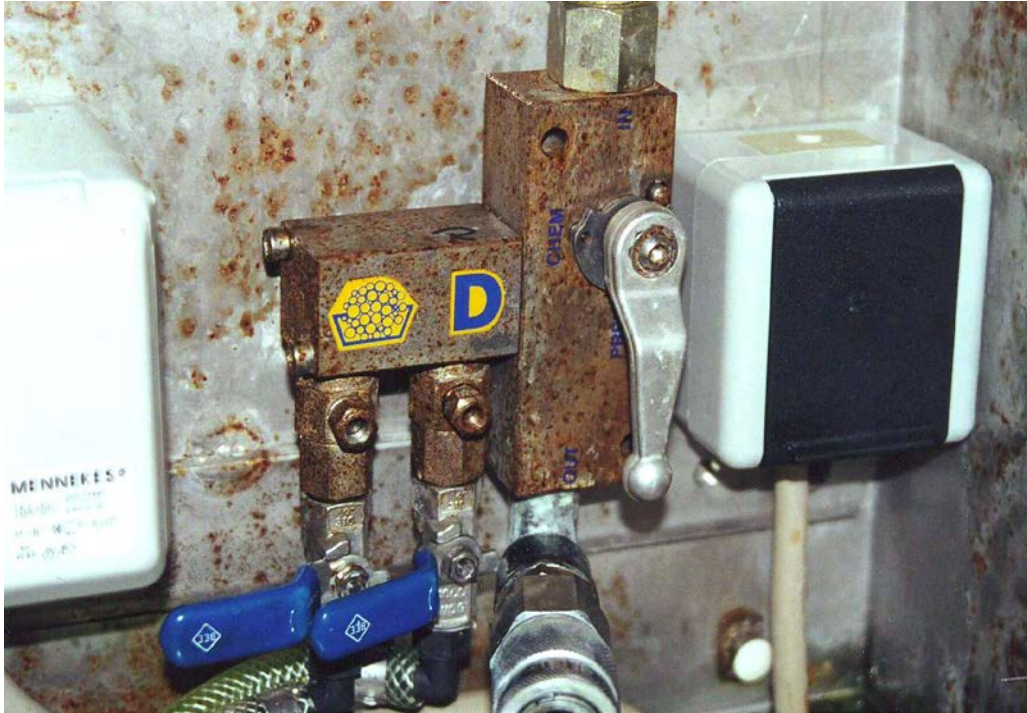
Fig. 8: Pitting corrosion and rust formation on fittings made of stainless steel 1.4301 in the technical room after 3 years
