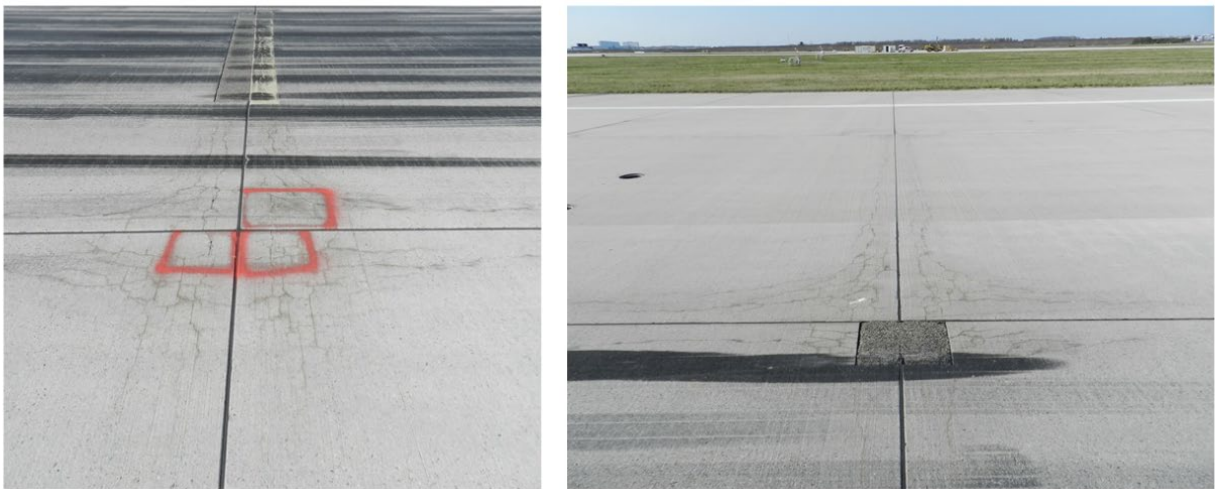
Fig. 1: Cracking following the perimeter of pavement slabs. Additionally the left figure includes the patching of the transverse joint and the right figure the patching of the corner
