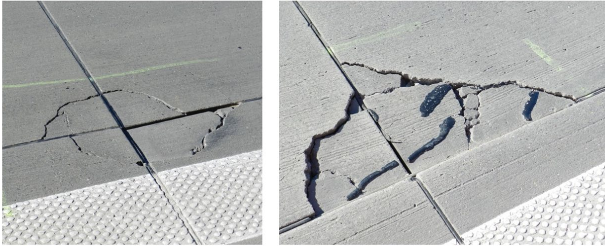
Fig. 6: Further deterioration, more cracking develops (left figure). Broken area may come loose (right figure)
