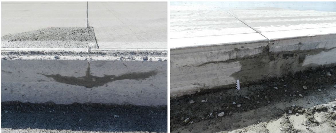
Fig. 3: Interior cracks parallel to the surface (left and right figure). In the left figure, the interior crack led to a corner crack, which had to be patched
