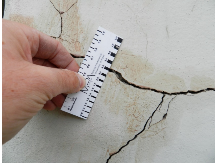
Fig. 7: Large cracks caused by ASR
