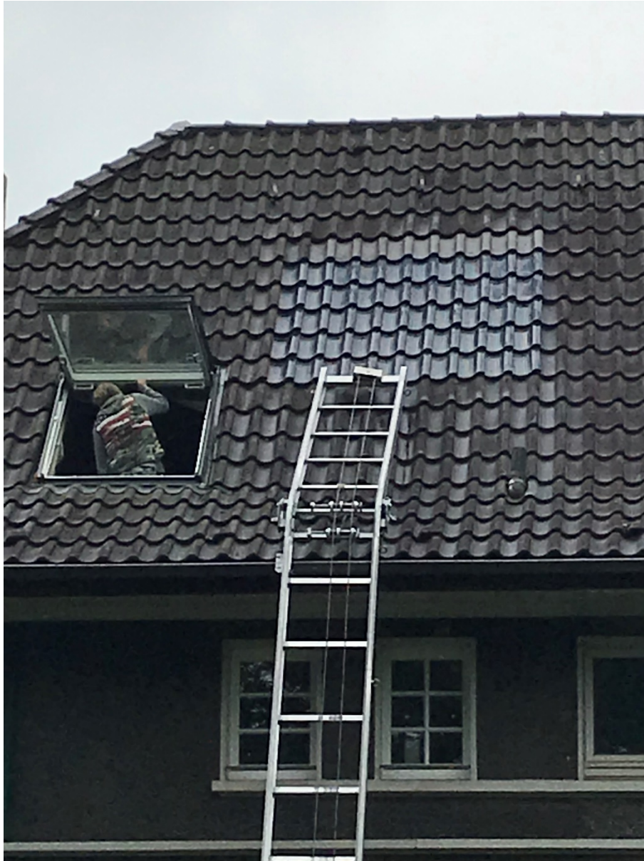
Fig. 5: View of the existing roof after replacement of the roof tiles by SHRT during sampling
