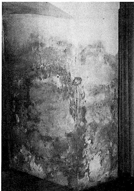
Fig. 1: A typical zone of rising damp, damaging the plaster and stone below and forming white efflorescences.
