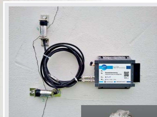
Instrumented crack monitoring with wire-less sensor nodes
